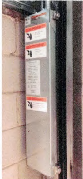
Transfer Switch Unit Mounted to Counterweight Guide Rail
