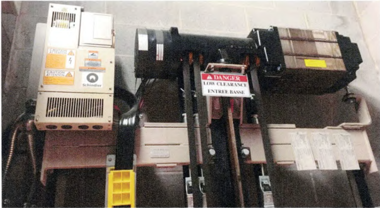
Equipment at the Top of the Hoistway
