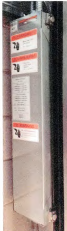
Transfer Switch Unit (TSU)
