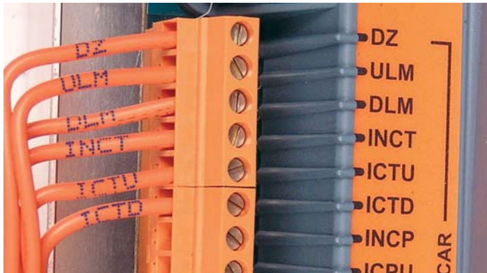
Typical label stamping at controller end
